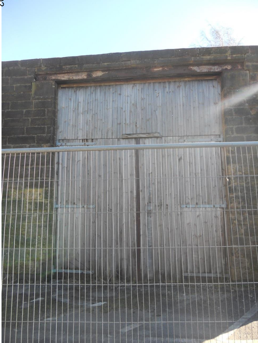
GOODS SHED DOORS WITH SAFETY FENCE
